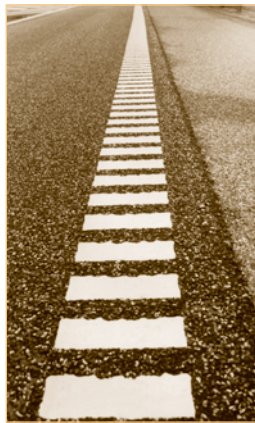
Visible Road Marking
